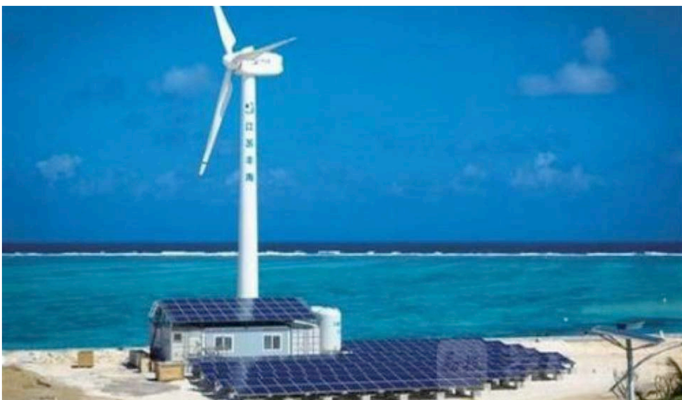
(Site photo of Desalination plant, wind & solar power combined equipment sets)
