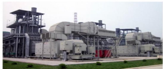
CONVENTIONAL COMBUSTION Up to 100% H 2
