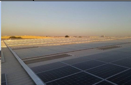
La Ronda Emirates Chocolate Factory, 649.6 kWp.
