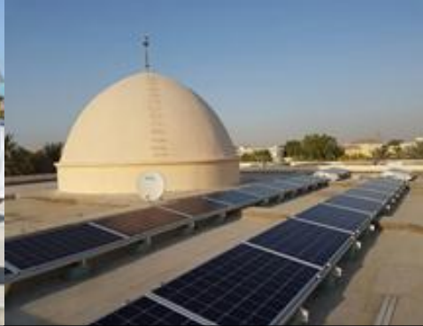
Awqaf & Minors Affairs Foundation (Mosque), Al Twar, 6 kWp
