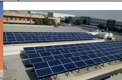
Royal Crown Fisheries Factory, 60 KWp
