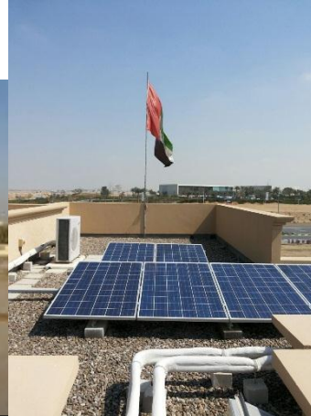
Private Villa, 5 kWp
